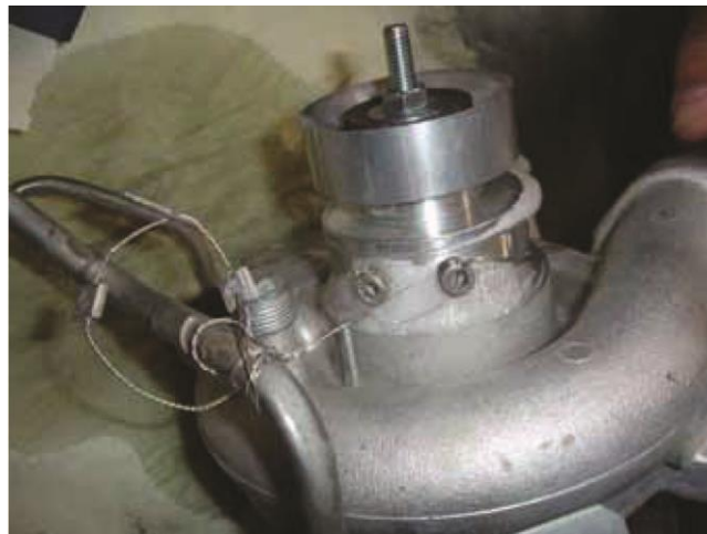
WRONG RESTRICTOR SEALING
